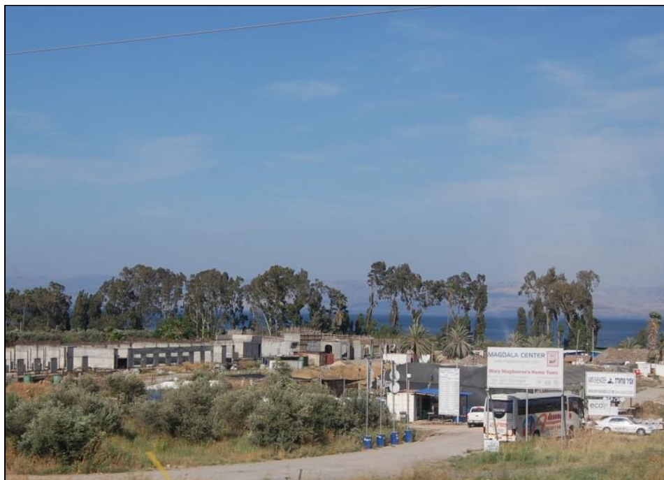
Early Construction of the Magdala Center with Black Canopies over the Synagogue
